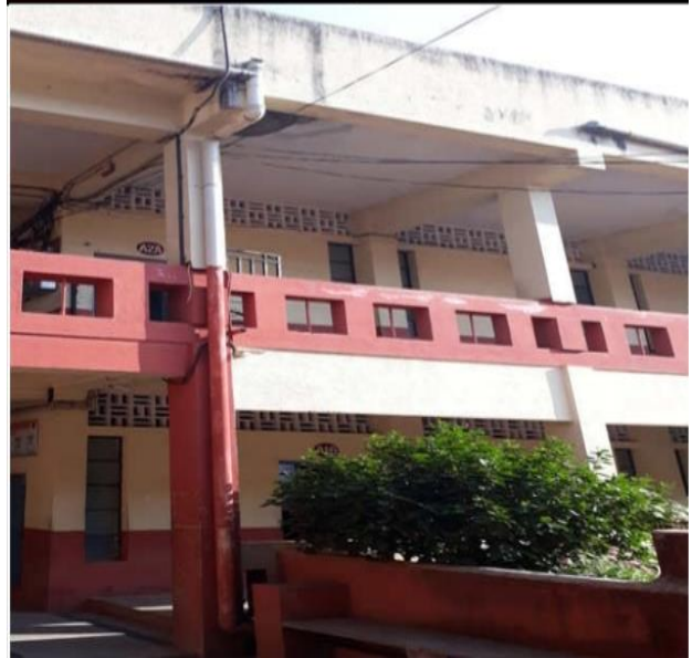
Active rooftop rainwater harvesting structure
